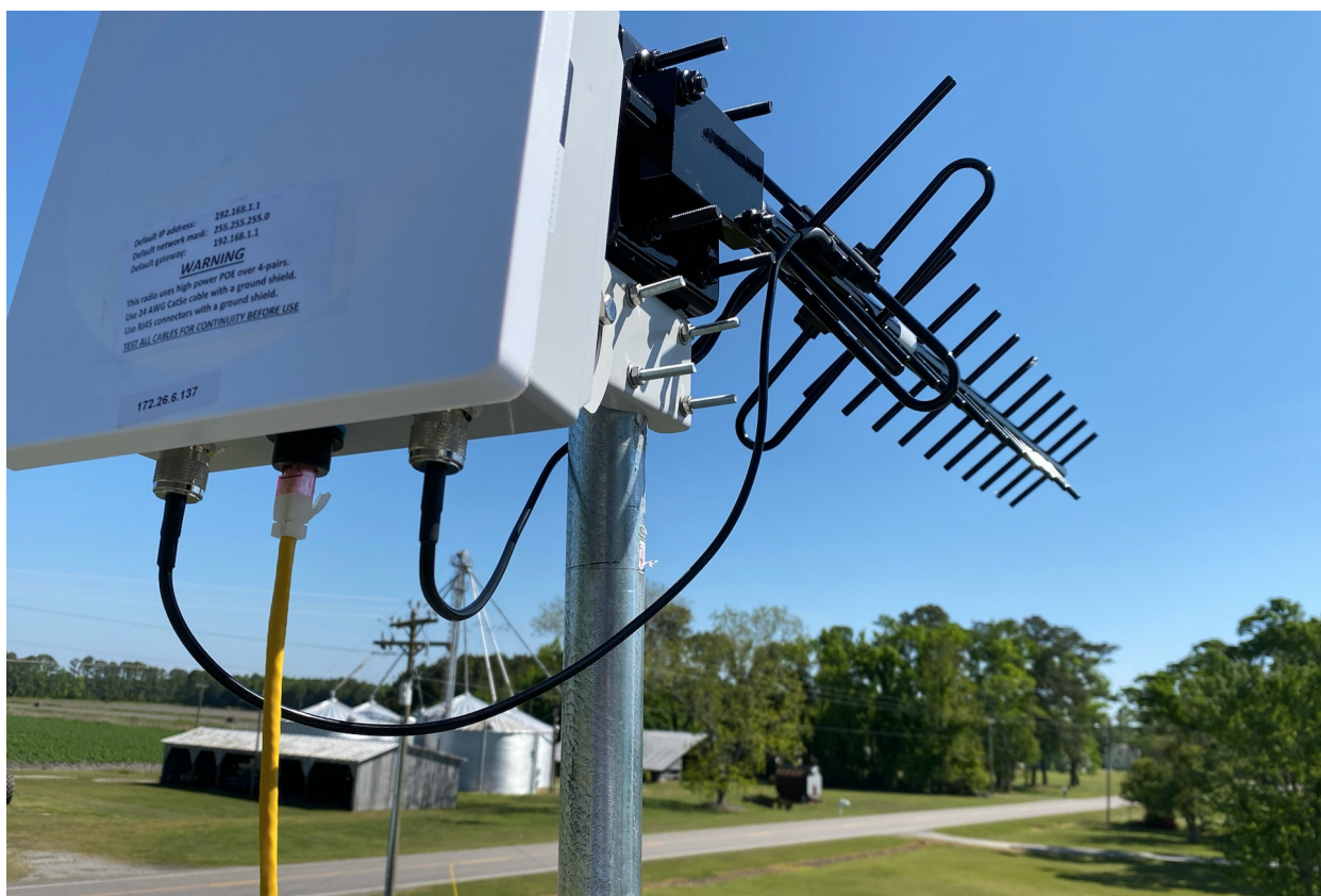
Figure 4. TVWS customer premises equipment installed near Engelhard, NC. Source: RiverStreet Networks)
