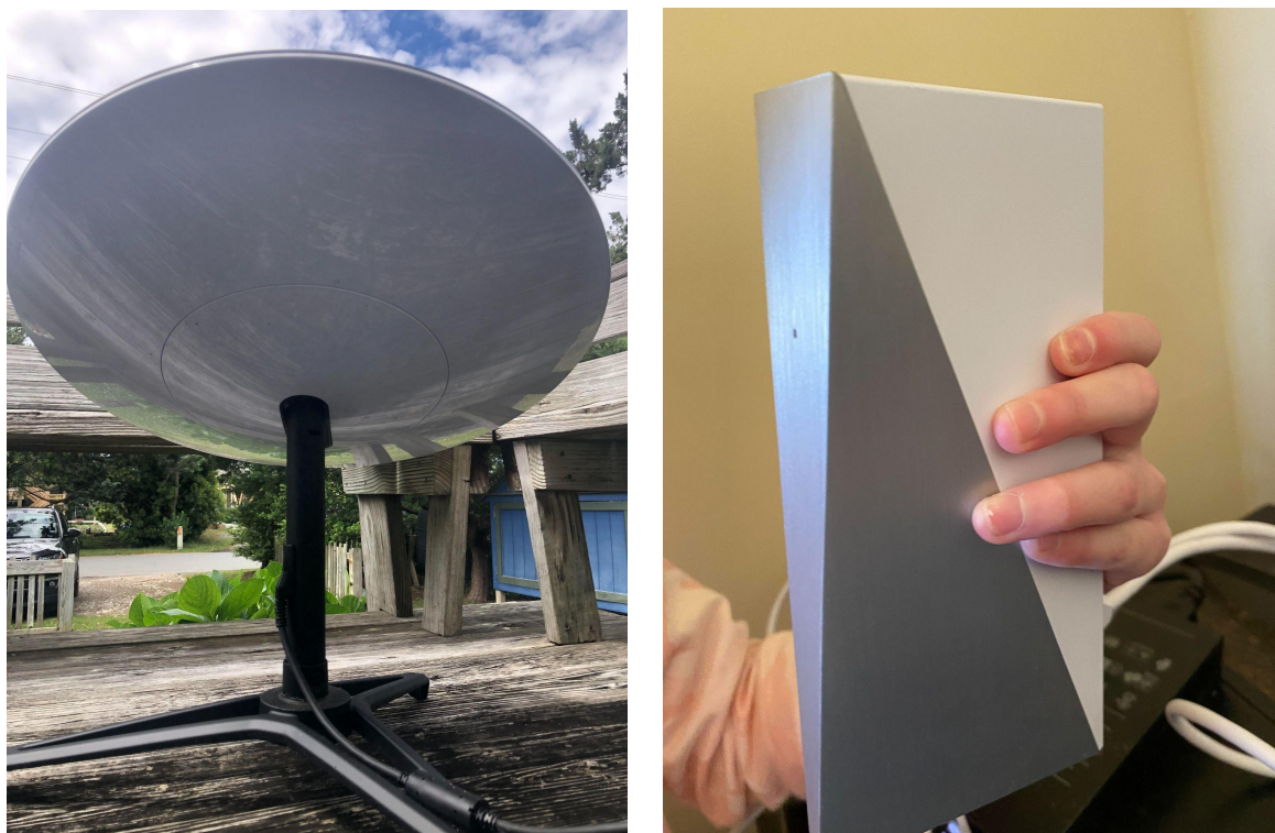
Figure 5. Starlink customer premises equipment installed on Ocracoke Island, NC. Left: Outdoor antenna. Right: Indoor Wi-Fi router. (Source: Hyde County Schools)
